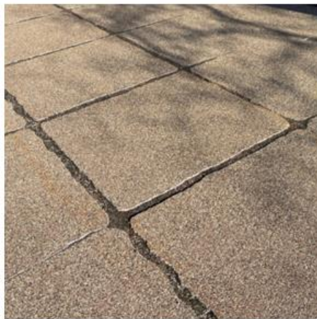
Wear on panel edges
