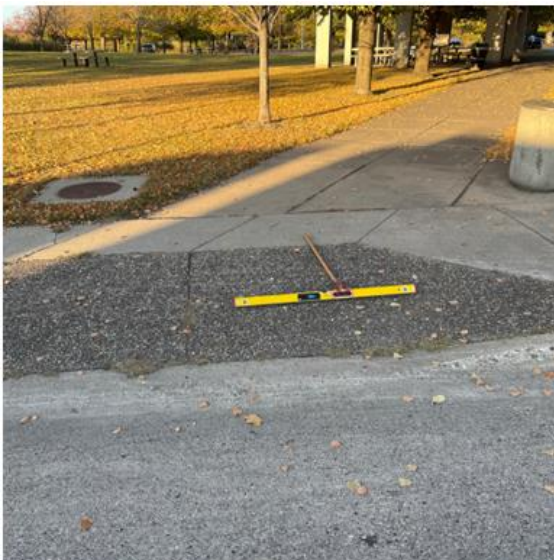
Non-Compliant Curb Ramp Without Truncated Domes
