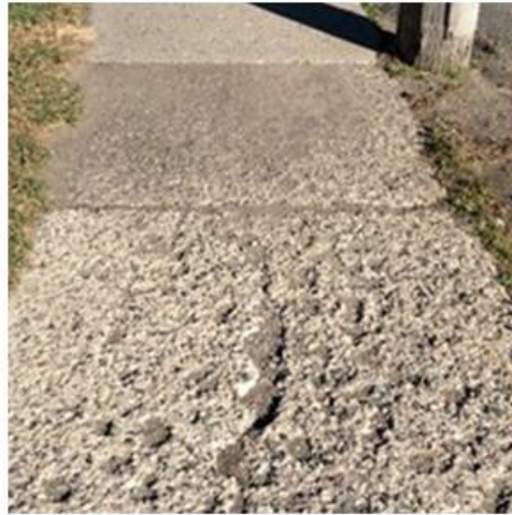
Surface wear and debris
